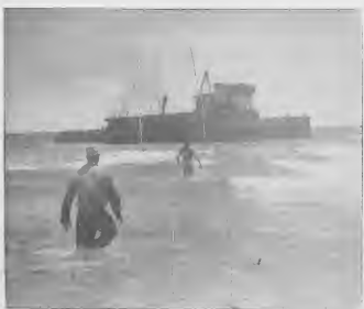
The Captain Rodger, a constant reminder of the ocean's power, may soon be demolished by men of the shipyard. The Rodger, wrecked when it attempted to aid a foundering superstructure is being removed (note that the stack is gone), although the job is made difficult by the heavy surf. Here, Welding Foreman Veri Clark (center) swims lines for the torches were stretched from shore to ship. Joseph Joseph, forecrafter, runs into the surf to grab a line washed sideways by the waves.
